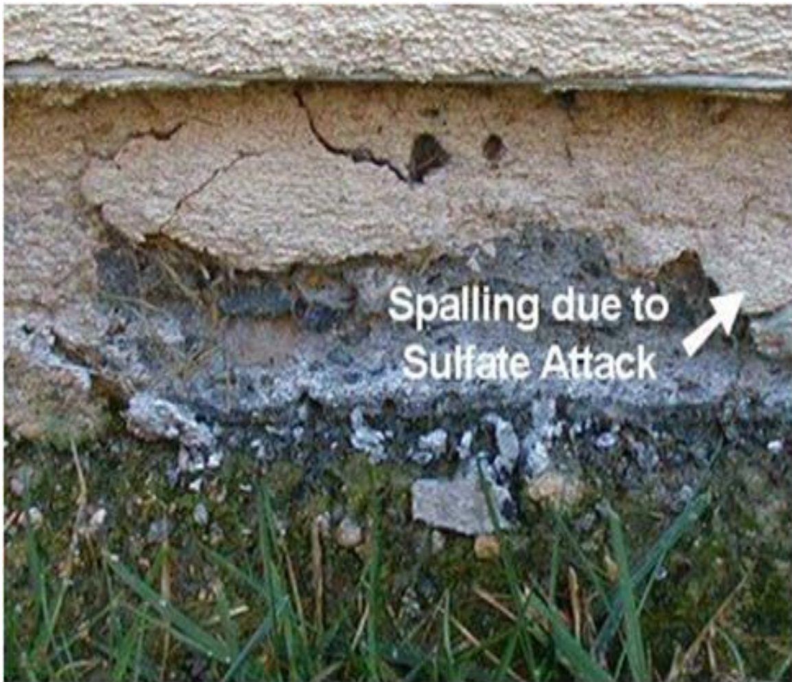
Figure 5 spalling due to sulfate attack [13] .
